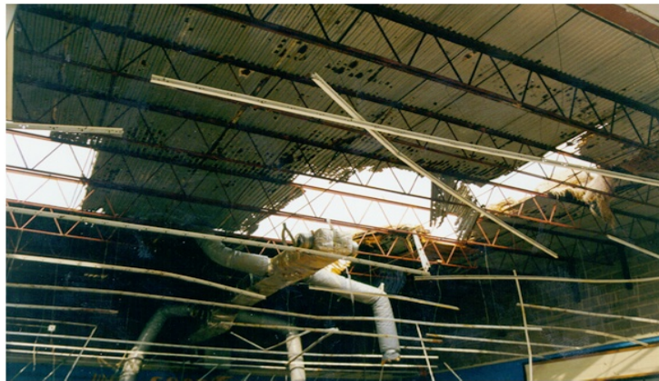
Figure 106. Wind Damage to a Roof Deck
