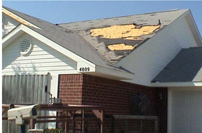
Figure 105. Wind Damage to a Roof Covering
