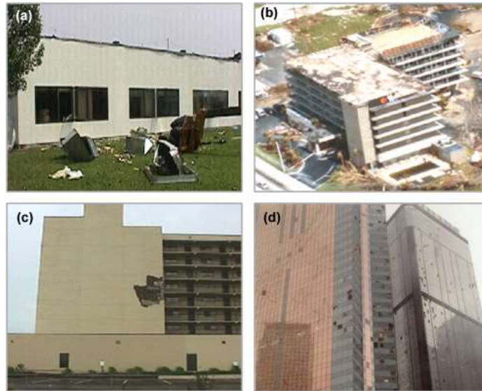
Figure 91. Damage to (a) Mechanical Equipment, (b) Roof, (c) Cladding, and (d) Windows
