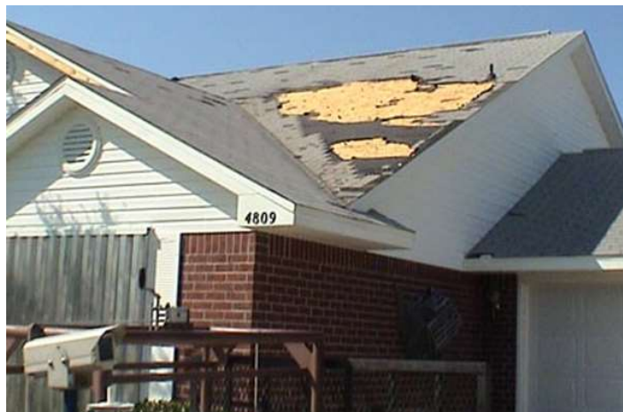
Figure 94. Wind Damage to a Roof Covering
