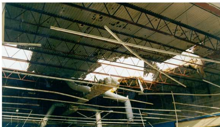
Figure 95. Wind Damage to a Roof Deck
