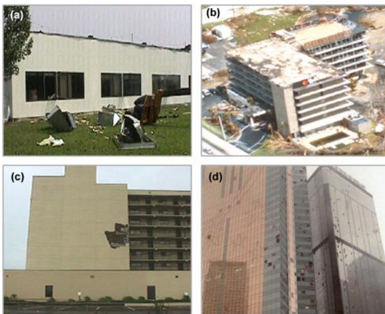
Figure 85. Damage to (a) Mechanical Equipment, (b) Roof, (c) Cladding, and (d) Windows
