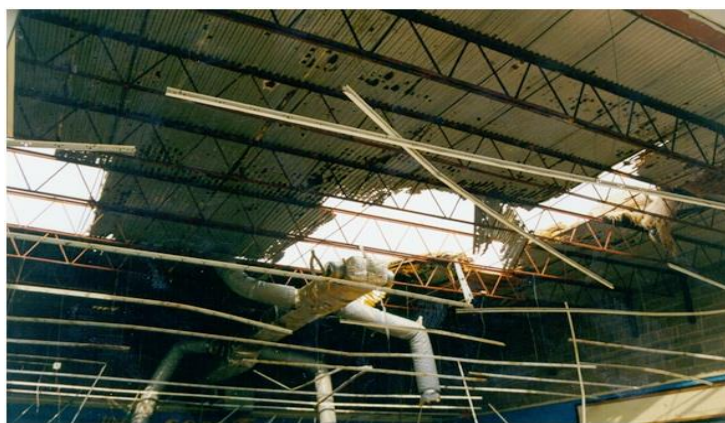
Figure 89. Wind Damage to a Roof Deck
