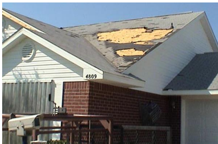
Figure 88. Wind Damage to a Roof Covering
