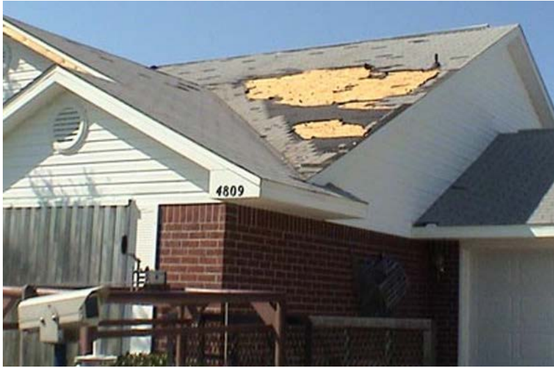
Figure 13. Damage to Roof Covering.
