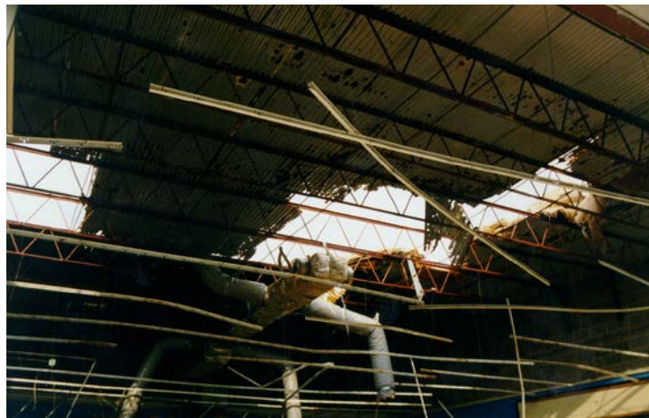
Figure 14. Damage to Roof Deck
